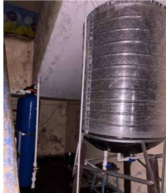
CMC R O Plant 500 LPH at Zilla Parishad Central Primary School, Valti, Pune
