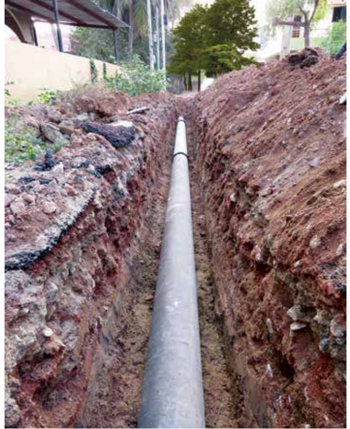
250 mm dia DI Pipe Laying at Balaji Nagar Zone at Dedicated Water Supply Scheme package-IV for Madurai Corporation in Tamil Nadu
