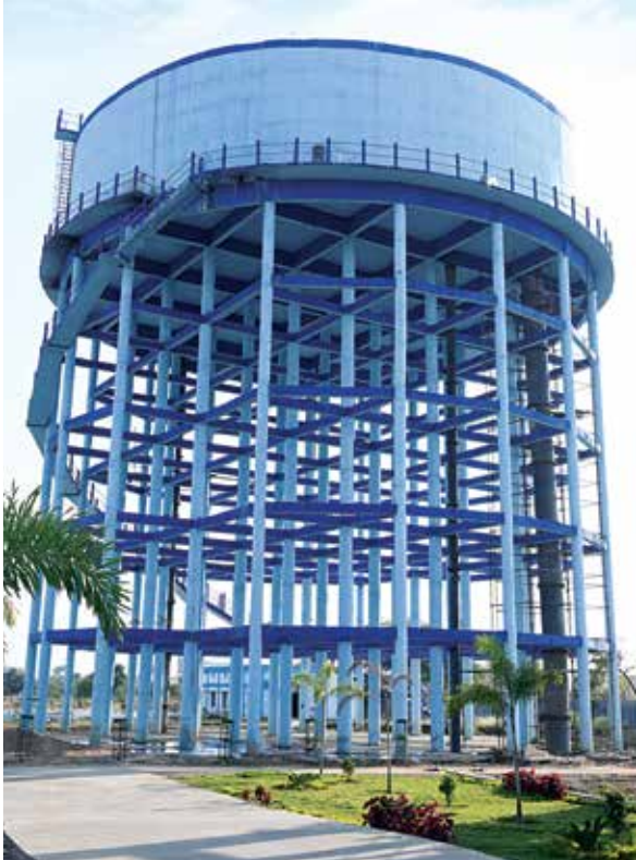
4680 KL Capacity of 25 Mtr staging Master Balance Reservoir at Bilaspur Water Supply Scheme in Chhattisgarh.
