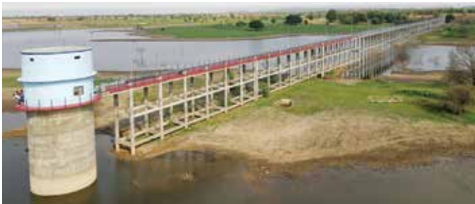
18.27 MLD of Intake Well cum pump house with Approach Bridge for a length of 630 meters for Gadakota Multi Village Rural Water Supply Scheme in Sagar District in Madhya Pradesh.
