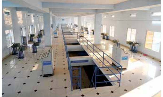
10 nos Filter bed in 72 MLD Treatment plant at Bilaspur Water Supply Scheme in Chhattisgarh.
