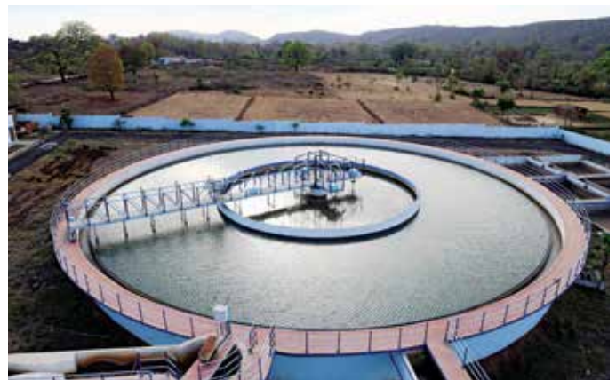
29.10 MLD Water Treatment Plant at Indwar Multivillage Rural Water Supply Scheme in Madhya Pradesh.
