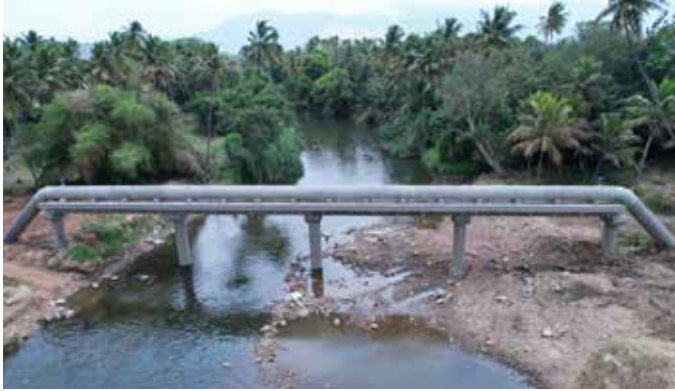
48 Mtr length RCC PCB across periyar river at Uthamapalayam of 1118 mm MS pipeline laying at Dedicated Water Supply Scheme package-I for Madurai Corporation in Tamil Nadu
