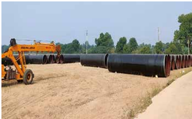
2028 mm dia MS pipe Stock Yard at Ramsan Village for Palanpur Package-ii project, in Gujarat.
