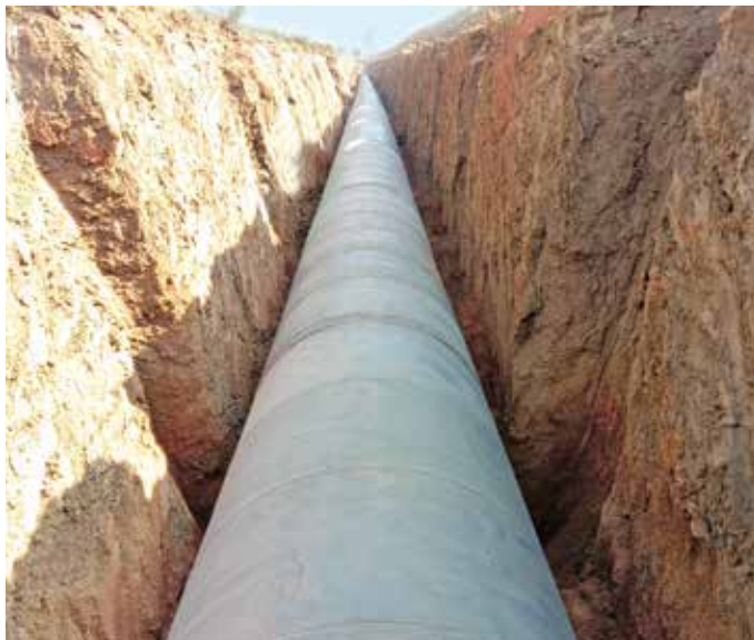
1500 mm dia MS pipeline laying at Bilaspur Water Supply Scheme, in Chhattisgarh.
