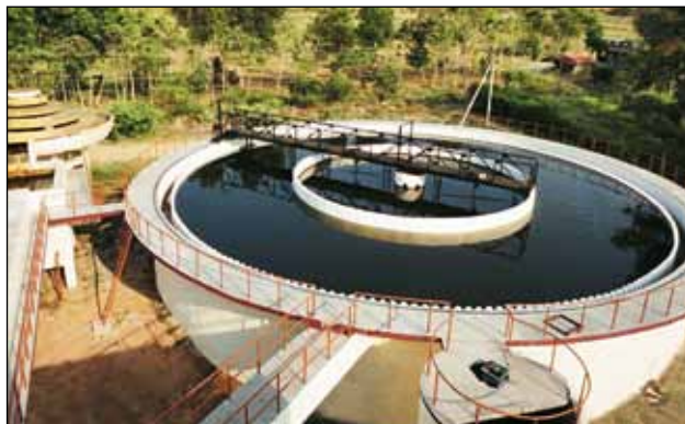
Construction of Aerator & Clariflocalator for 11.75 MLD water treatment plant under the work of CWSS to Madathukulam & other 112 Rural Habitation of TWAD Board, Coimbatore
