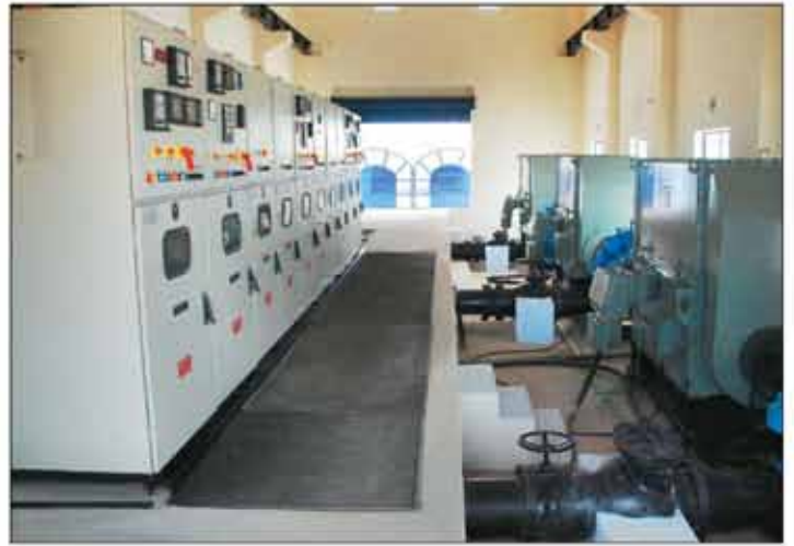
Pumps and Motor
