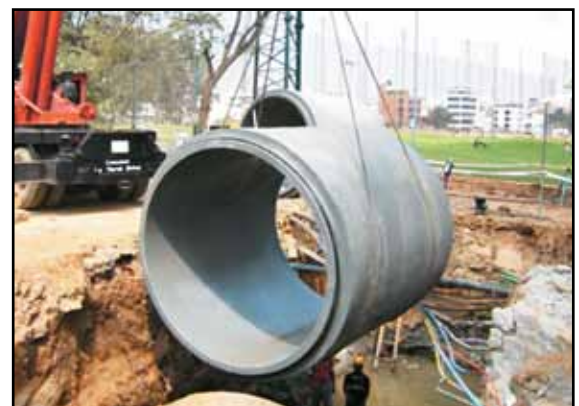
2400 mm dia R.C.C. NP-3 class pipe with polyurea lining for the sewerage work contract S2B for BWSSB, Bangalore
