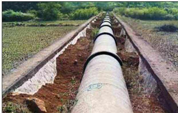
1100 mm dia PSC Pipe line for Vadiwale Left Bank Canal pipe line project Near Pune, Maharashtra
