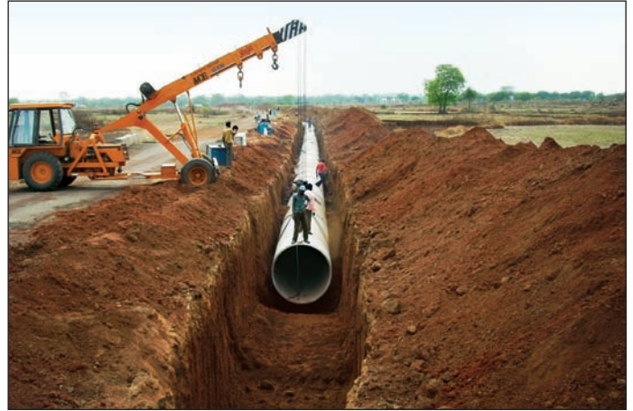
1700 mm and 1400 mm dia M.S. Pipeline for Raipur Augmentation Water Supply Scheme.
