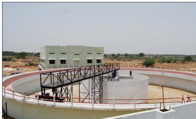
Clarifloculator at Gajwel Phase-I Project.
